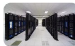
Data Center Monitoring
