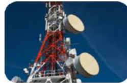
Telecom Tower Remote Monitoring
